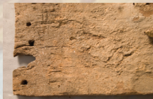
Fig.8: Decayed wood and dowels hole in the side wood board
